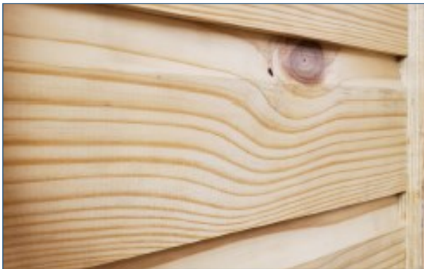
Figure 162: Unpainted wood siding.
