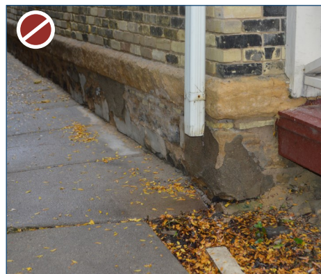
Figure 127: Improper drainage gutter system resulting in deterioration of foundation walls.
