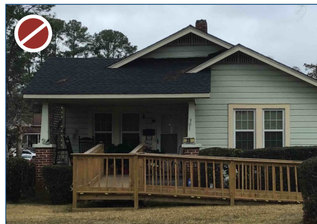
Figure 88: Inappropriate ramp installation on the front façade of a residential building.
