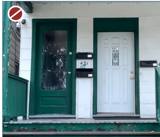
Figure 104: Inappropriate replacement of a historic door (right door).
