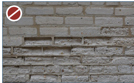
Figure 94: Inappropriate modern mortar replacement on a historic building resulting in damaged bricks.
