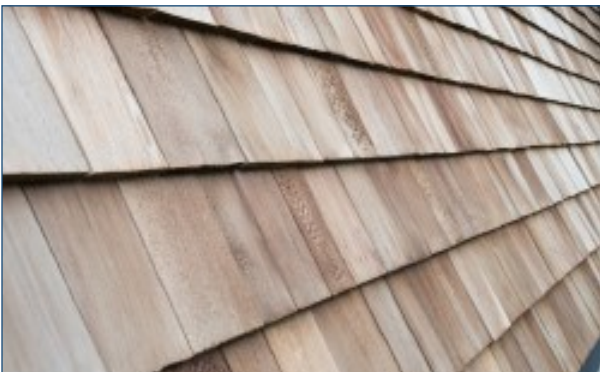
Figure 163: Unpainted wood shingles.
