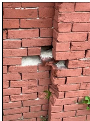
Area of Damaged Brick/Masonry
