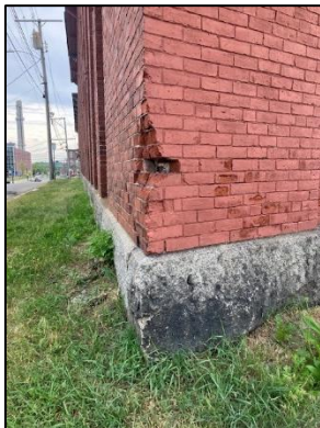
Area of Damaged Brick/Masonry
