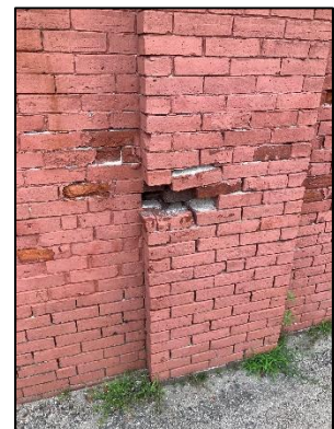
Area of Damaged Brick/Masonry
