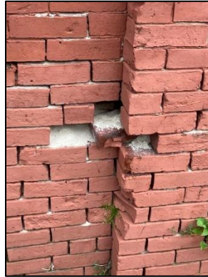
Area of Damaged Brick/Masonry
