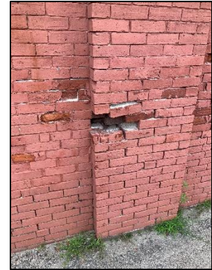
Area of Damaged Brick/Masonry
