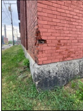
Area of Damaged Brick/Masonry
