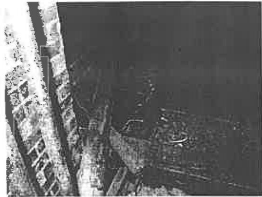
Hole in attic floor
