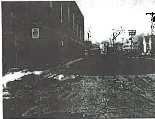
Entrance to north parking area showing poor condition of pavement
