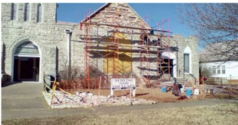
Figure 11: View showing the selective demolition at the south gable before re-setting of the blocks occurred, 2015. Stonefell Chapel (website).
