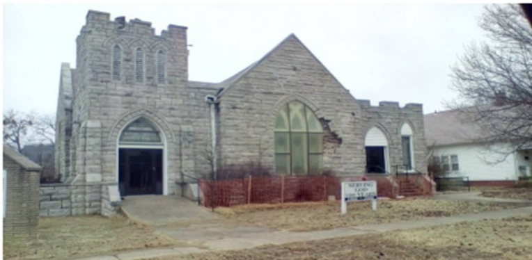
Figure 10: View showing the delaminating stone wythe at the south gable, 2015. Stonefell Chapel (website).
