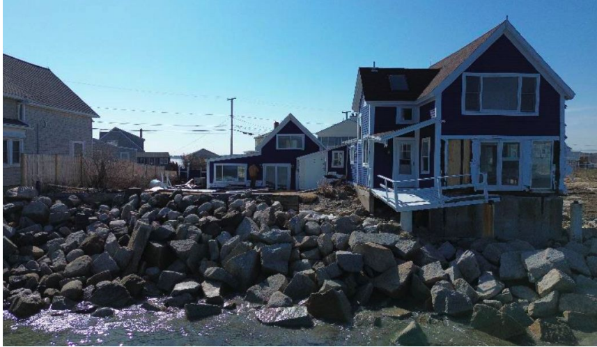
Wrap around deck destroyed, porch roof unsupported. Photo taken from Forensic Engineering Solutions report, dated March 11, 2024
