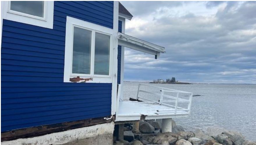
Wrap around deck destroyed, porch roof unsupported.
