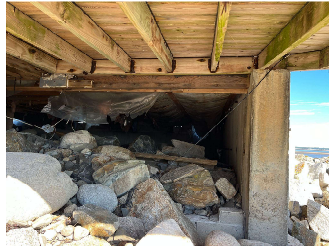
Existing foundation wall missing, sea wall infiltration
