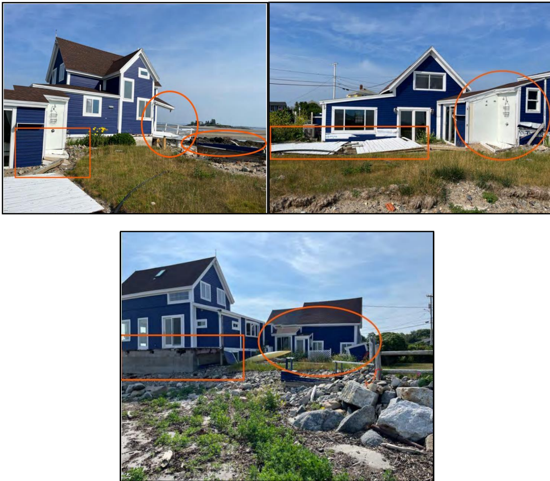
Figure 4 Further damage to the property that was sustained by the January storms.
