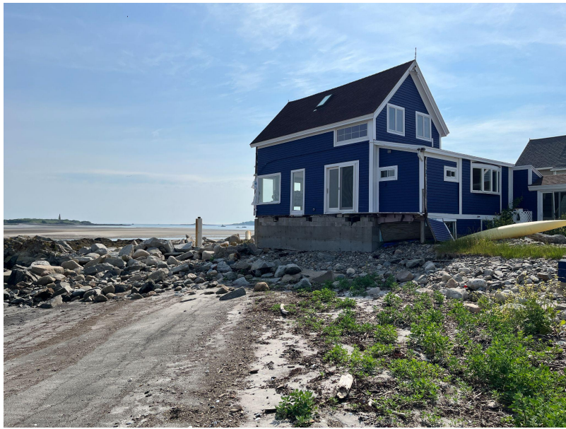
Wrap around deck destroyed & damage to existing foundation wall.
