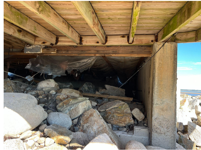
Existing foundation wall missing, sea wall infiltration
