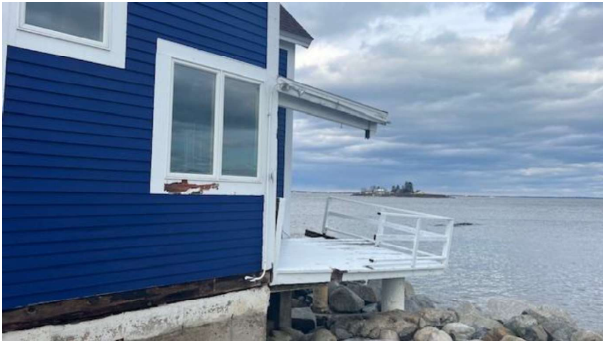
Wrap around deck destroyed, porch roof unsupported.
