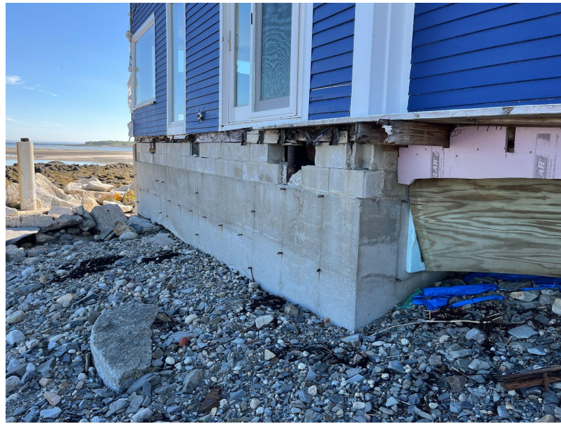
Missing CMU and cracks in west foundation wall.
