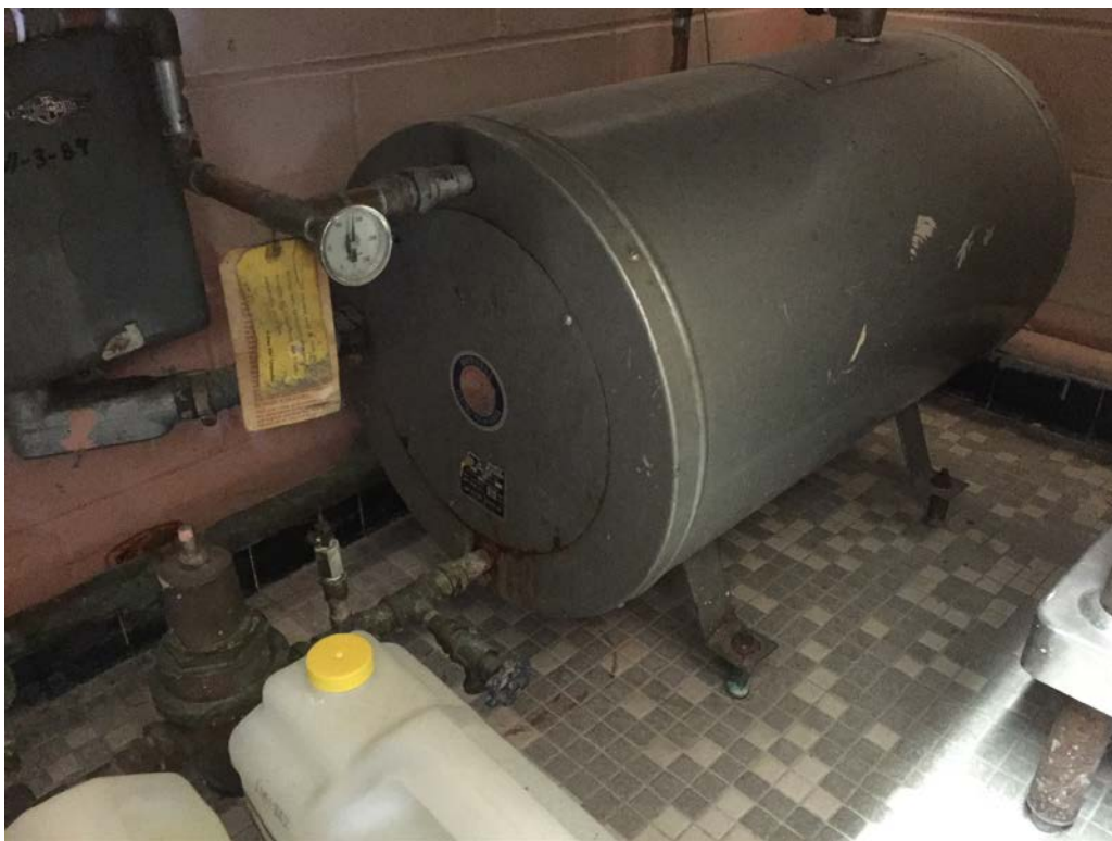
Plumbing Photo 1 – Electric booster water heater.
