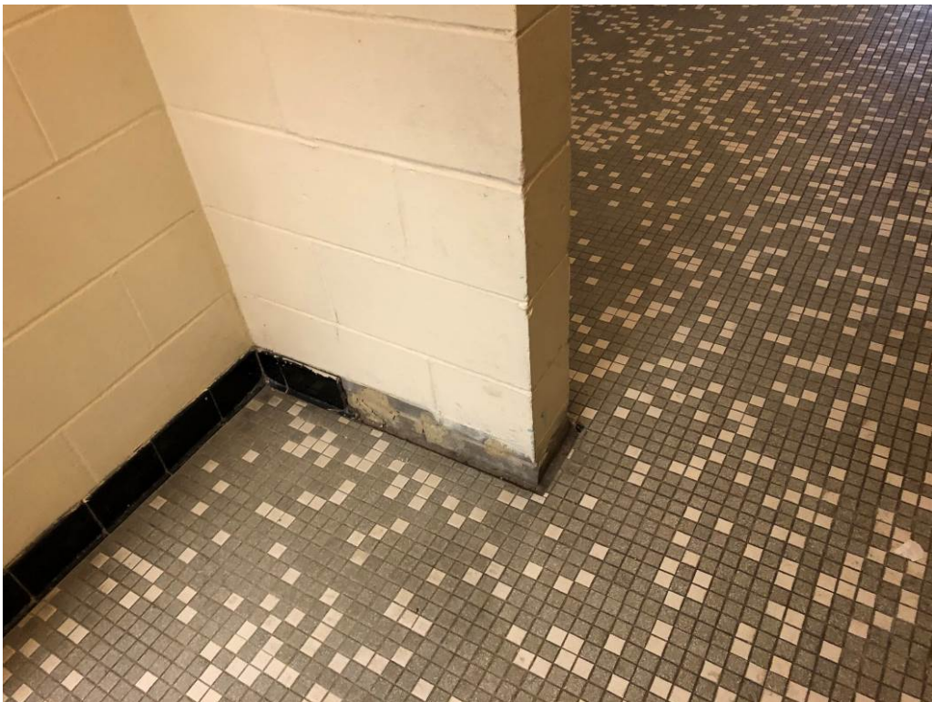
Architectural Photo 14 - Typical multi-user toilet room floor.
