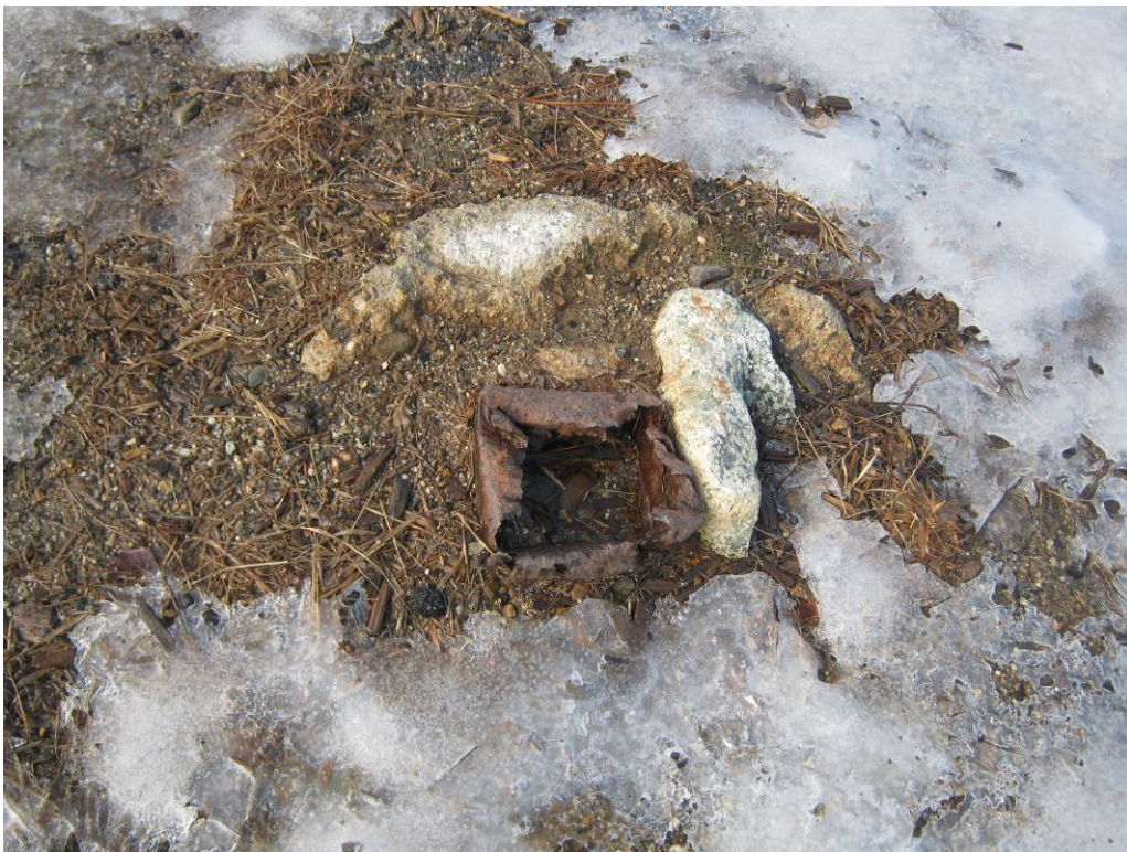
Civil Photo 32 - Sheared-off post and concrete base at playground.
