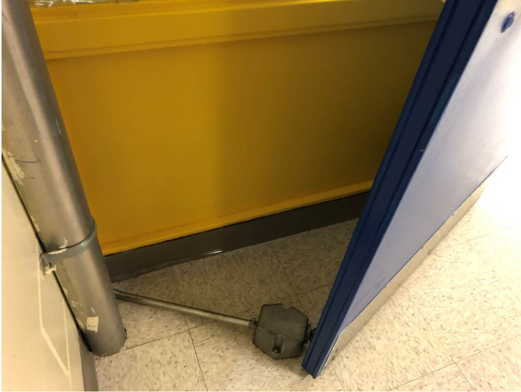
Architectural Photo 17 - Electronic magnetic door holder, typical at all stairwell enclosure storefronts.
