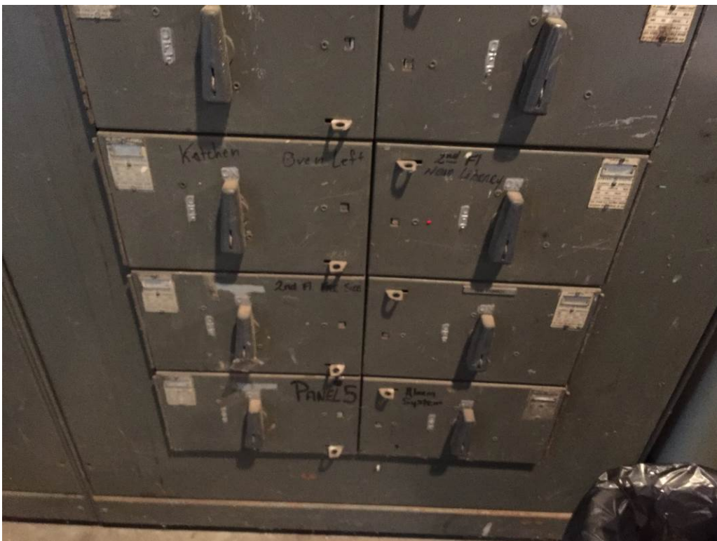
Electrical Photo 1 - Main distribution panelboard.
