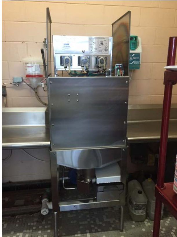
Mechanical Photo 3 – Commercial dishwasher.
