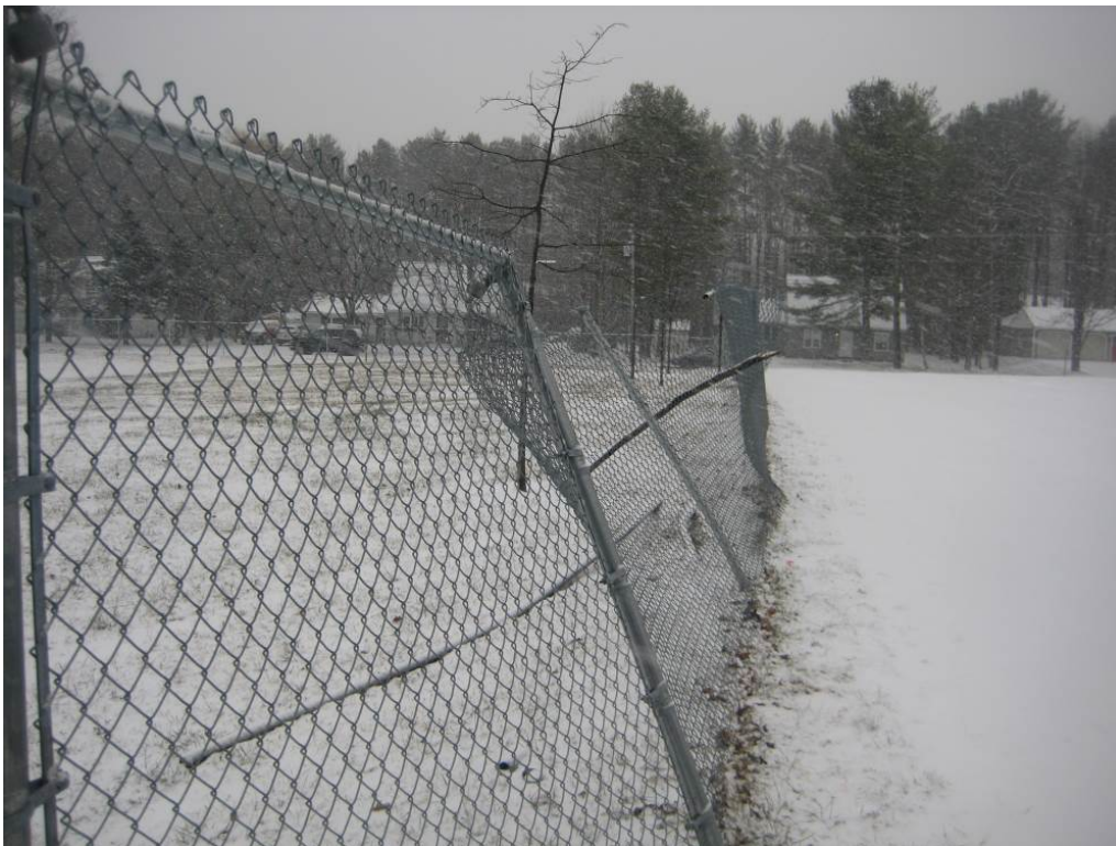
Civil Photo 18 – Damaged chain link fence near vehicular access to the playground on western side of site.
