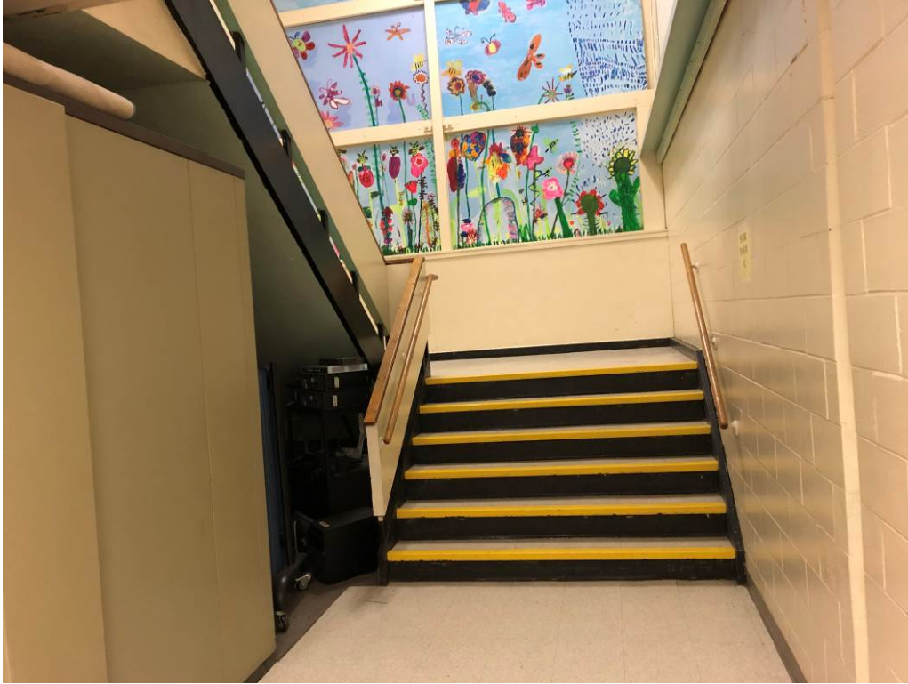
Architectural Photo 9 - Stair 2 showing overall condition, non-complaint handrails, guardrail, riser and tread.
