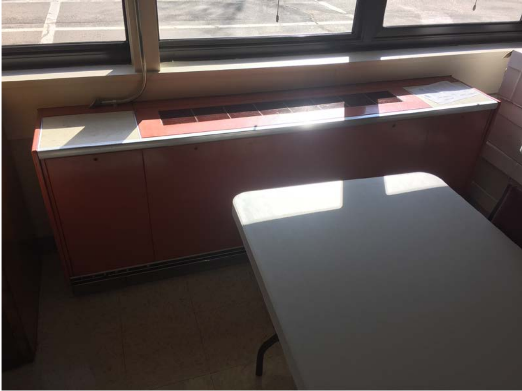
Mechanical Photo 1 – Typical unit ventilator.
