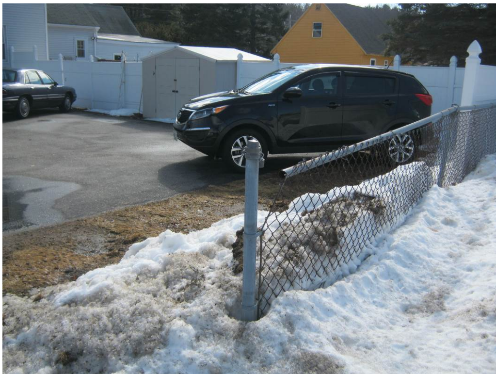
Civil Photo 16 - Chain link fence in poor condition.
