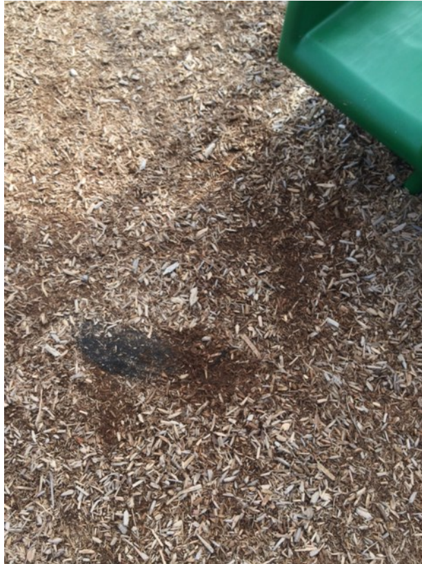
Civil Photo 29 - Geotextile fabric exposure at playground.
