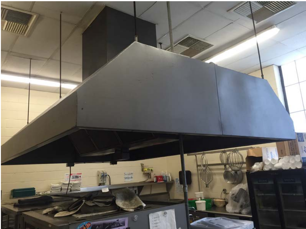
Mechanical Photo 2 – Kitchen exhaust hood.
