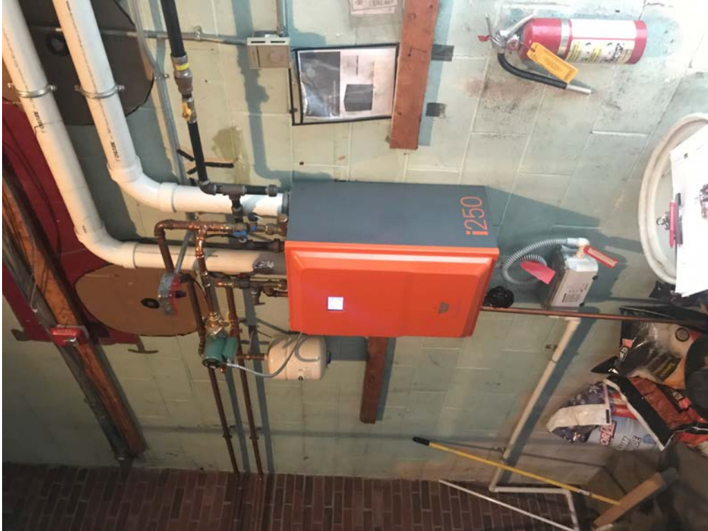
Plumbing Photo 2 – Gas-fired water heater.
