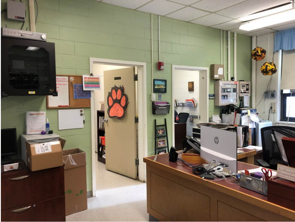
Architectural Photo 5 - Typical condition of admin offices with non-ADA complaint door hardware.
