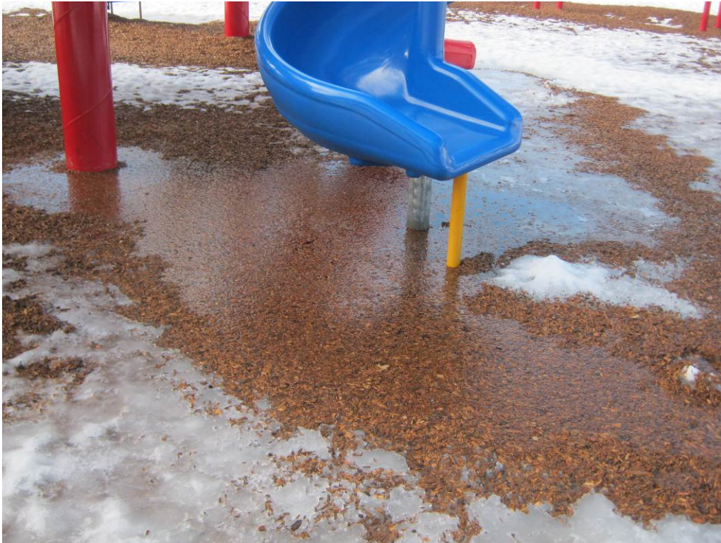
Civil Photo 25 - Water ponding at base of slide.
