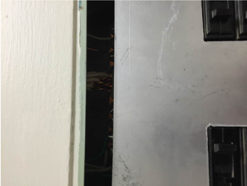
Electrical Photo 2 - Branch panelboard with exposed wiring.
