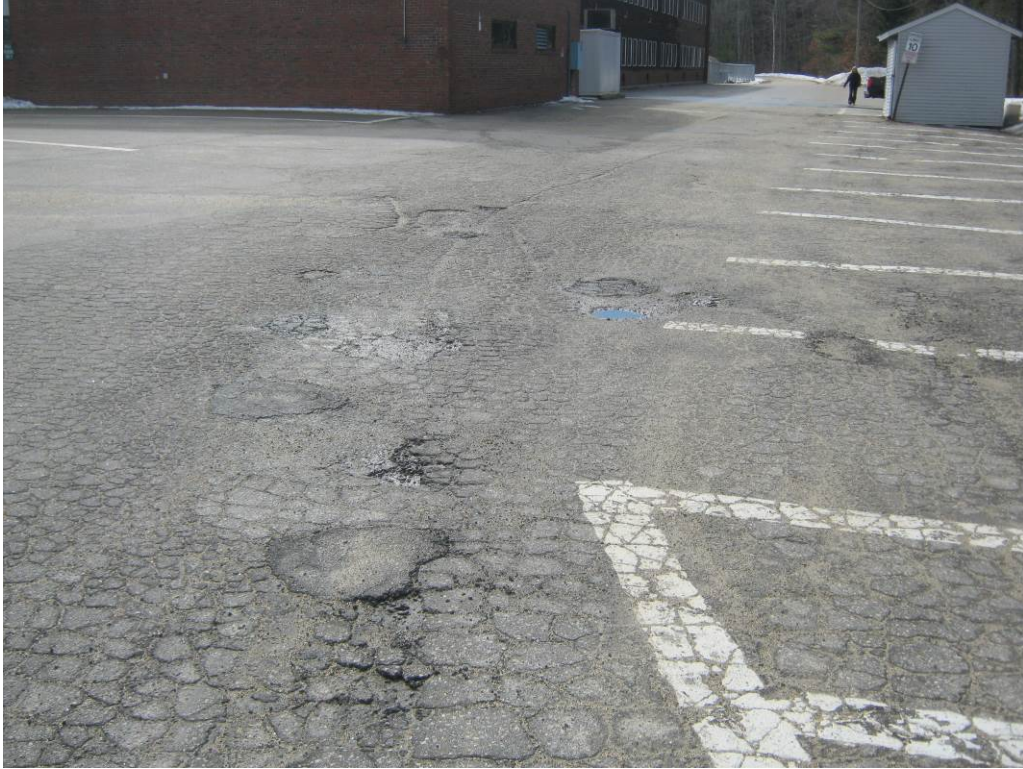
Civil Photo 9 - Pavement in poor condition.
