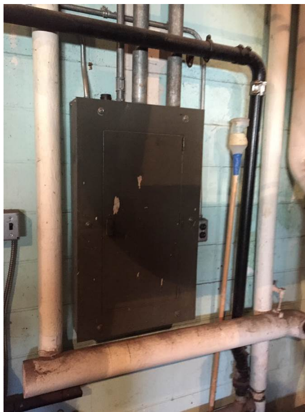
Electrical Photo 3 - Branch panelboard with pipes located within dedicated equipment space.
