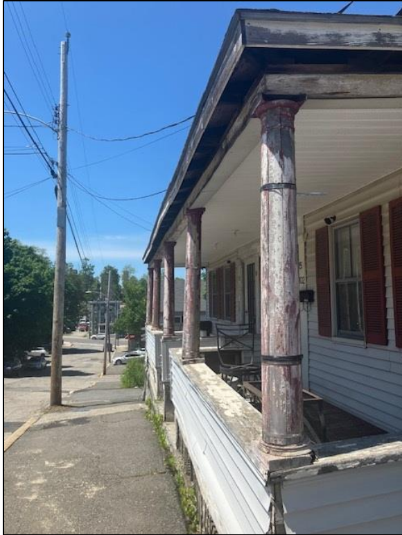
The existing columns are splitting vertically and are held together by hose clamps.
