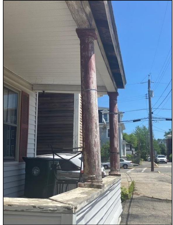
The front of the porch is leaning outward severely.
