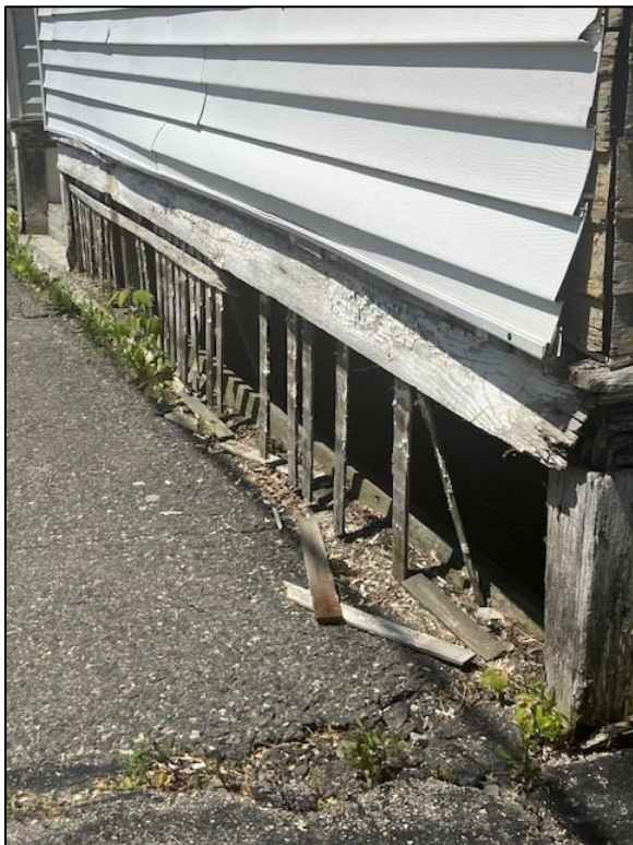
Much of the structure is rotting.
