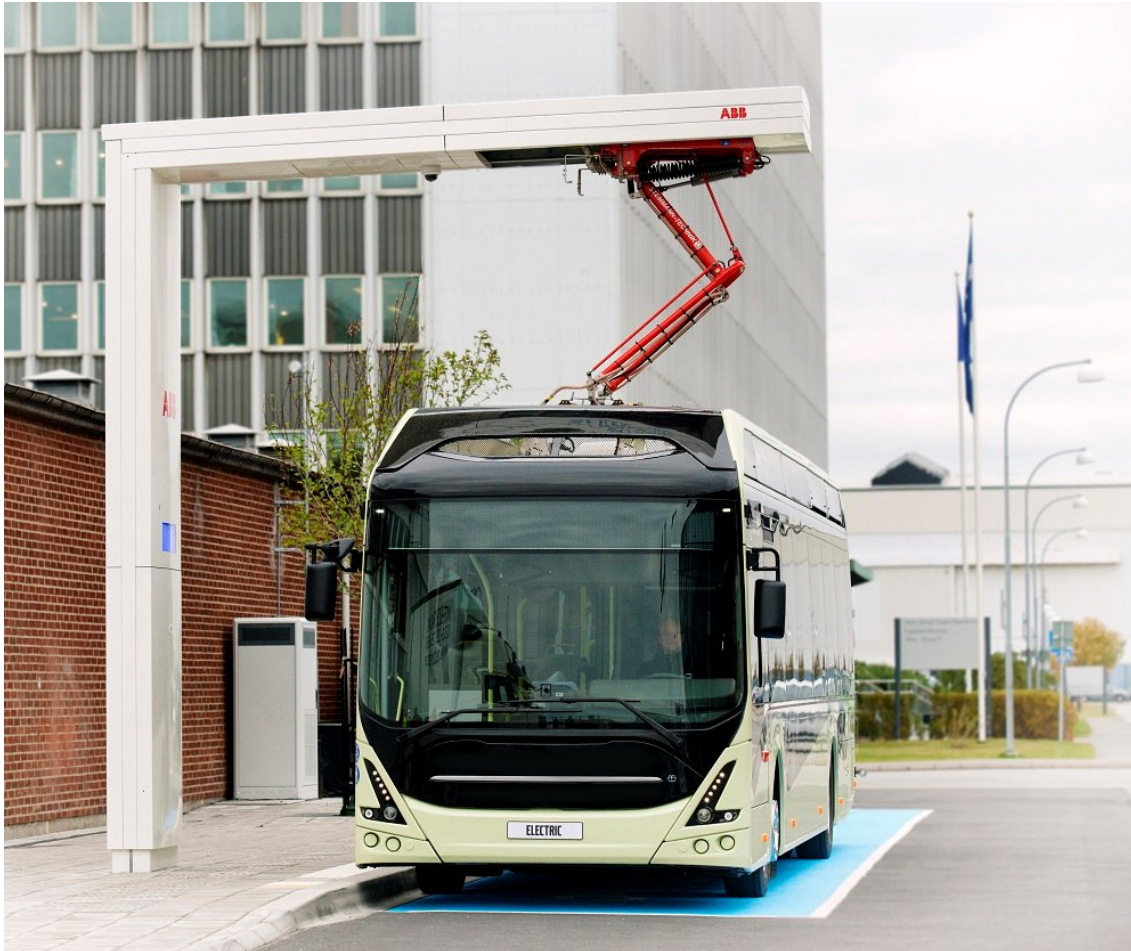
Charging infrastructure example.
