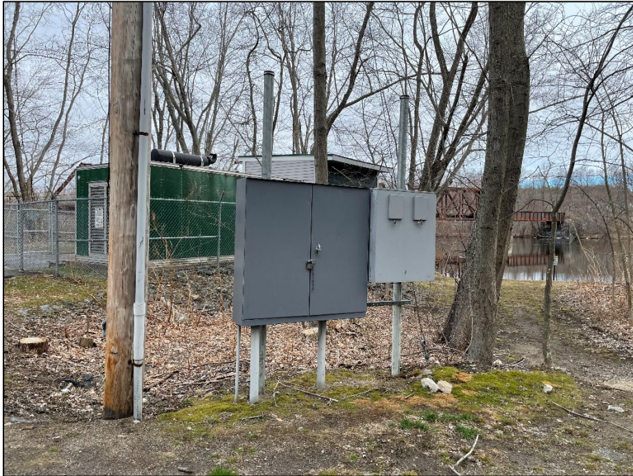
Photo 5: Existing electrical panels, to be demolished
