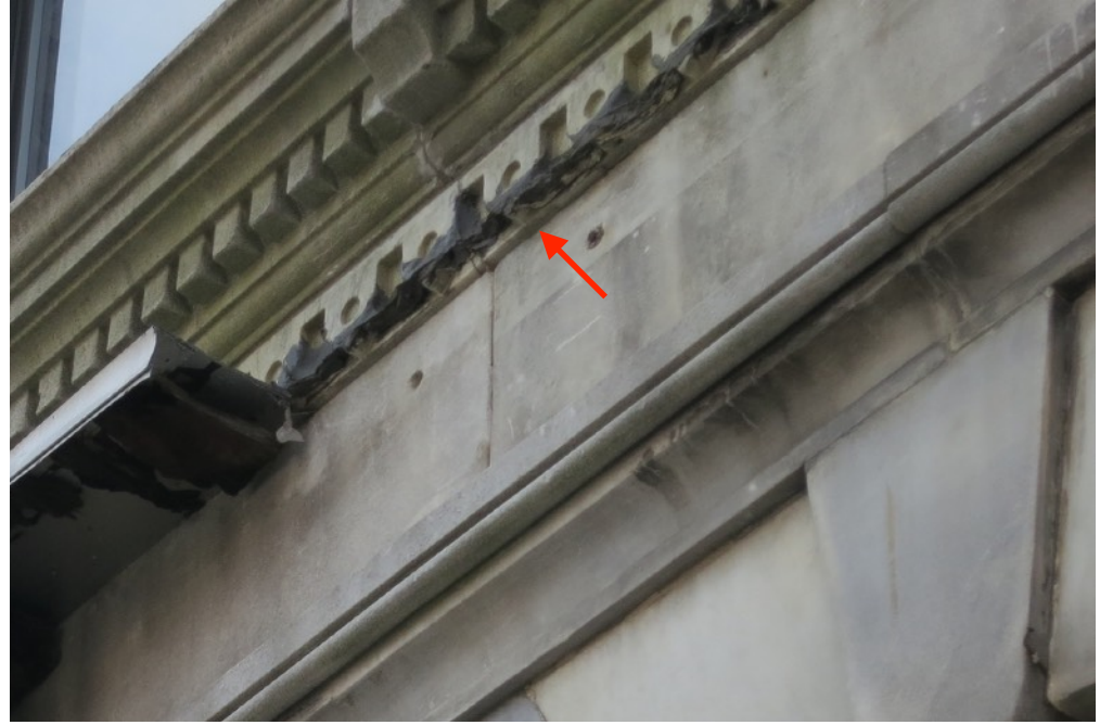
74 | Detail at facade showing remnants of bituminous caulking
