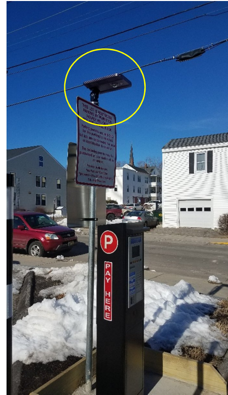
Figure 2 - Solar Light Installation
