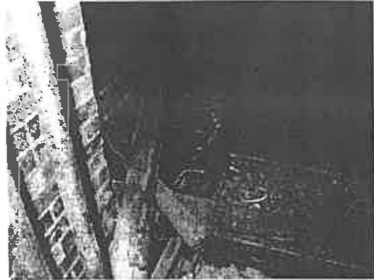
Hole in attic floor
