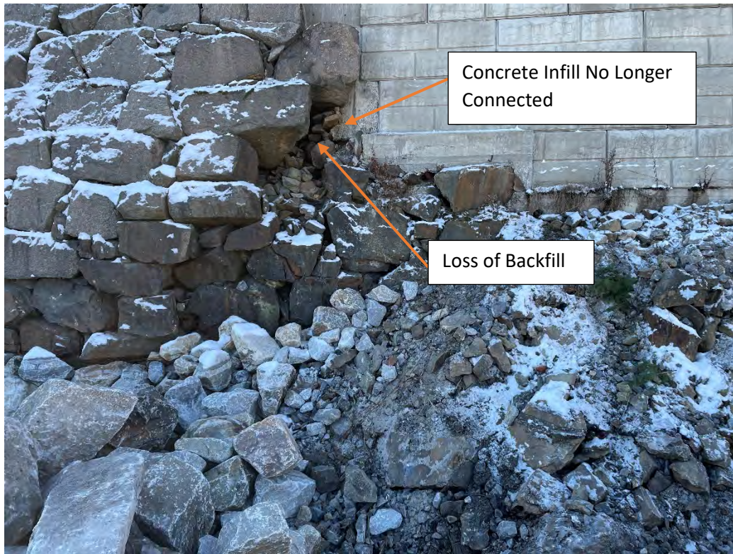
Photo 11 – Damage to East Side of MSE Wall, December 9, 2021
