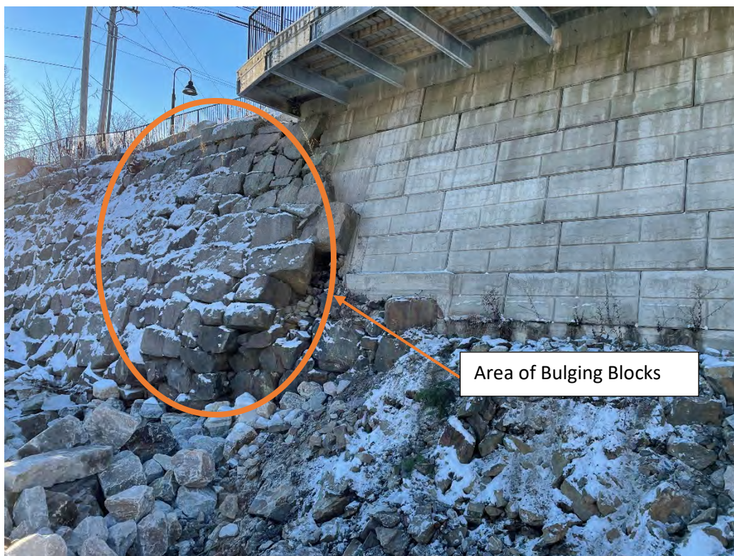
Photo 12 – Bulging of Stacked Block Wall, December 9, 2021
