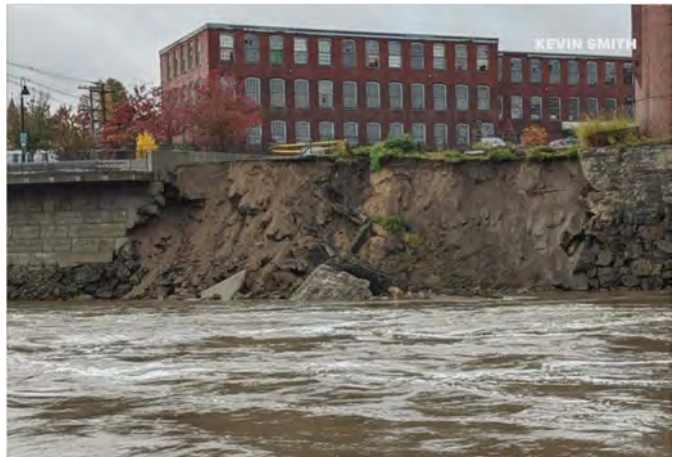
View of wall failure on November 1, 2021
