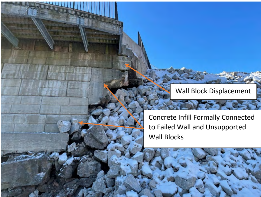
Photo 10 – Damage to West Side of MSE Wall, December 9, 2021
