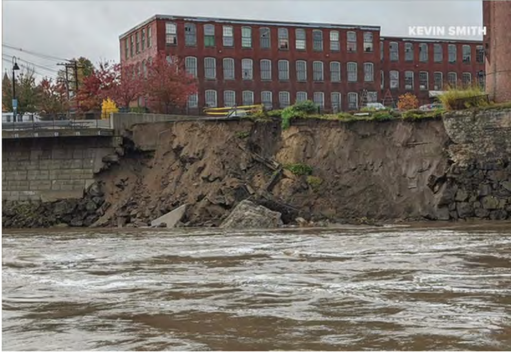
Photo 5 – Wall Failure Before Stabilization on about November 1, 2021
