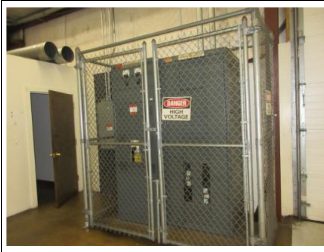
43) One of the main electrical entrances
