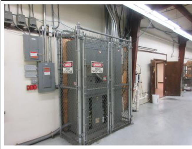
31) One of the main electrical entrances
