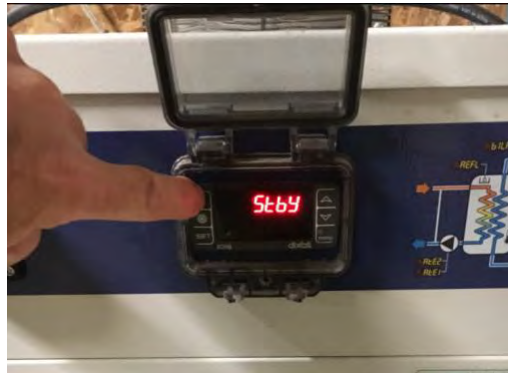
Chiller on STANDBY
