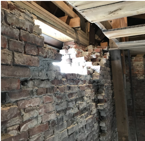
Masonry Before Repair
