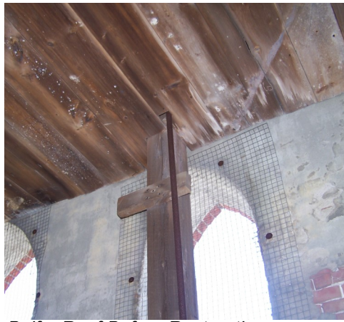
Belfry Roof Before Restoration
