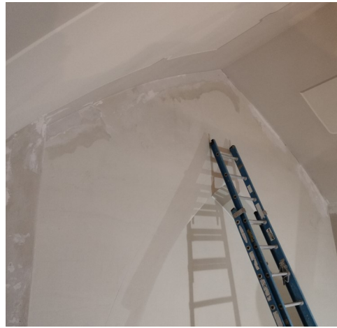
Plaster Before Repair
