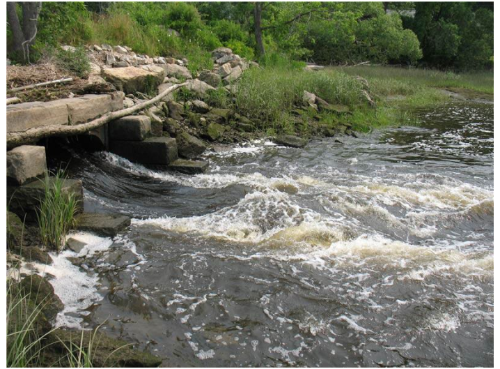
Existing undersized culvert
