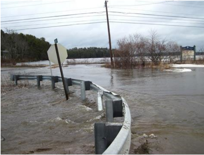
Recurring flooding at Rte. 1/George Wright Rd.
