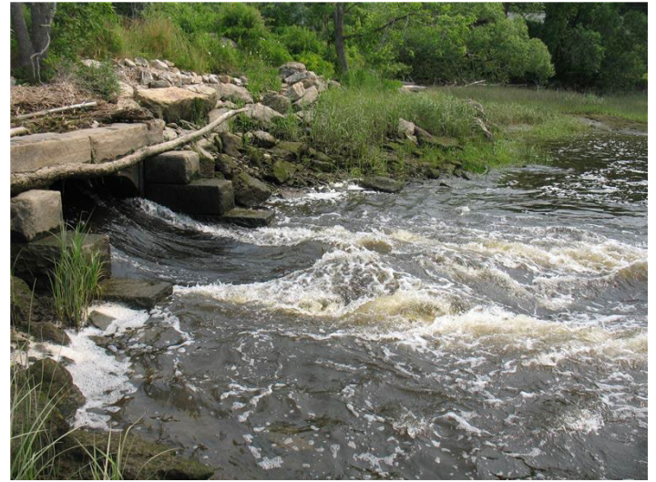
Existing undersized culvert
