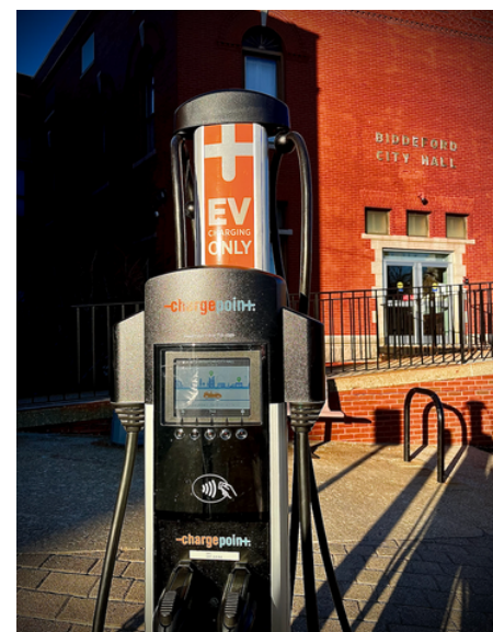
EV Charing Station. PhotoVoice Contest 2023 Entry.
