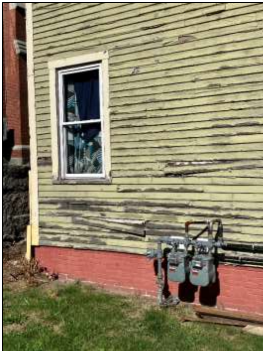
Southeast side with damaged areas
