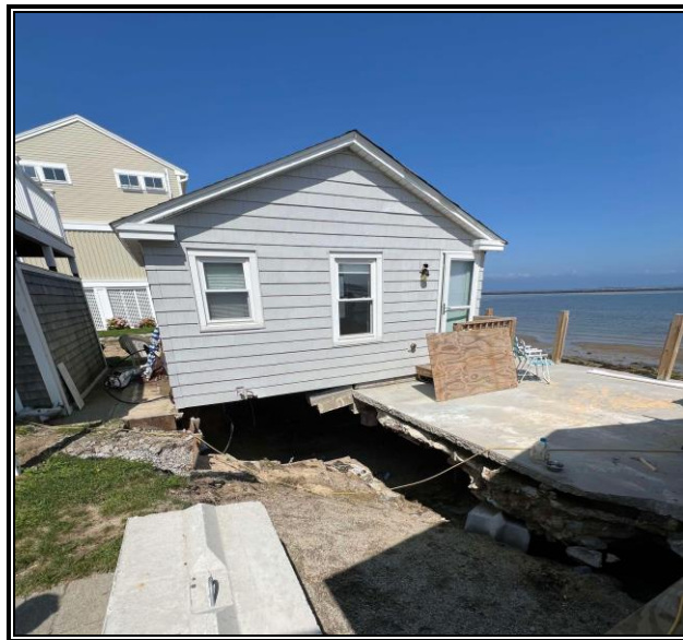
Figure 2: An illustration of the existing failed foundation
