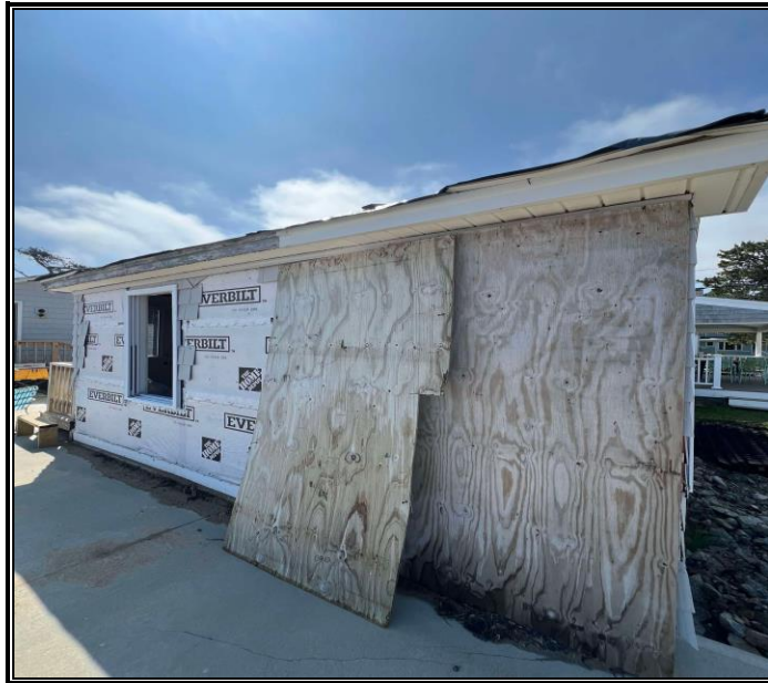
Figure 3: Exterior damage sustained as a result of the water.
