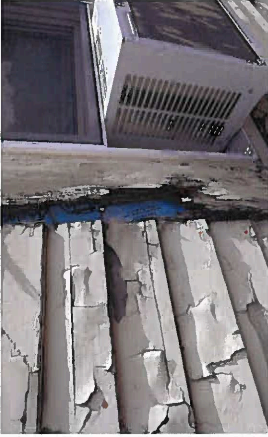
10 | Facade (south elevation) - water damage at first floor
