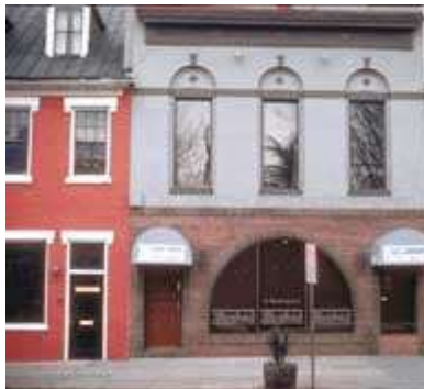
Incompatible replacement storefront and inappropriate window alteration.
