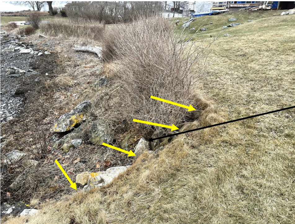
Shoreline erosion, roots of shrubbery exposed to air.
