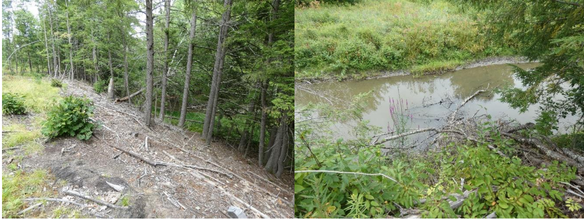
Figure 7. A narrow, forested buffer along Thacher Brook showing cut stumps on a steep bank (left) and a location where felled trees left no forested buffer at all along Thacher Brook (right). (Waypoints#1000 & #006)
