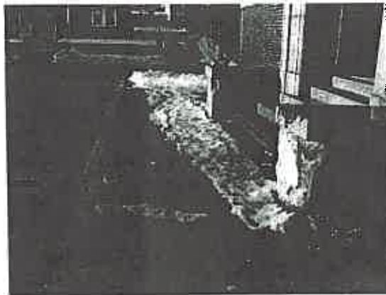
Deteriorated pavement and curb at southwest entrance
