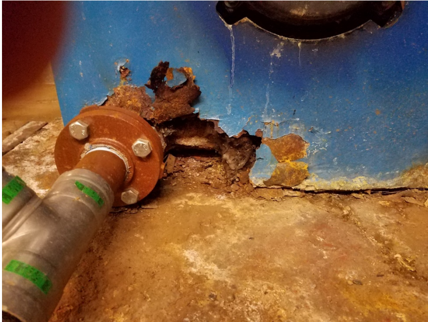
Picture #1 – View of Boiler at Point of Failure
