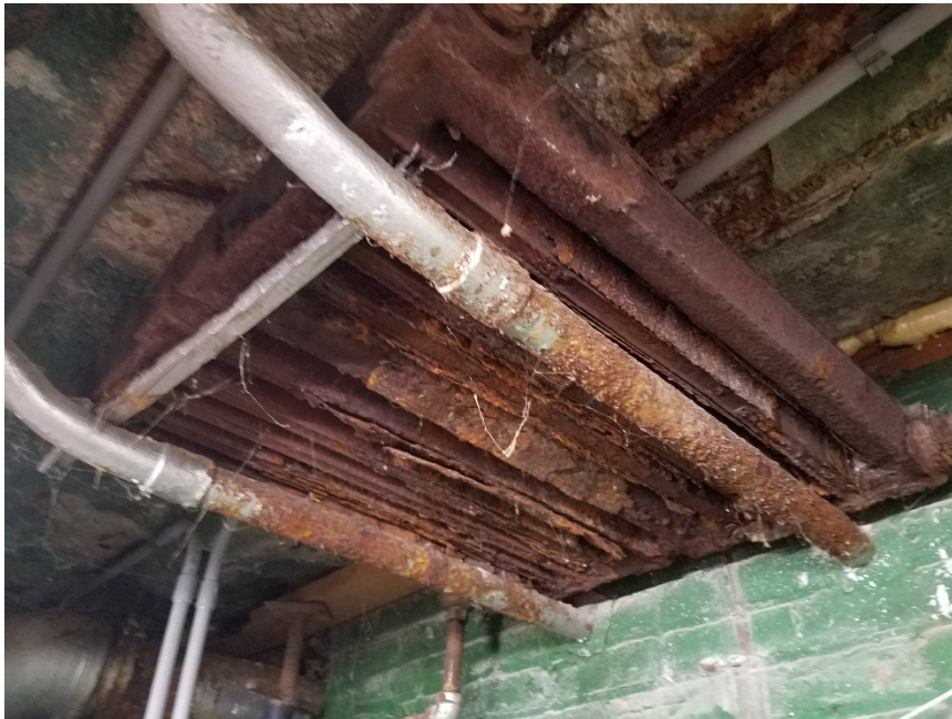
Picture #2 – View of Ceiling Radiator Corrosion
