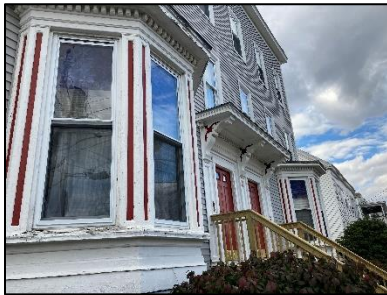
Above: Front bay windows. Rotted wood will be replaced.
