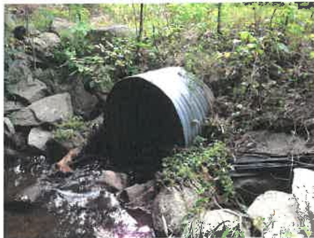
View of Culvert #1. This structure only passes approximately 50% of the natural channel width.
