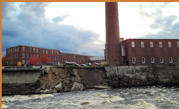
In 2021, an intense downpour washed out a large portion of an embankment along the Saco River in Biddeford, with repair costs estimated over $2 Million. Credit: A. Sherwin
