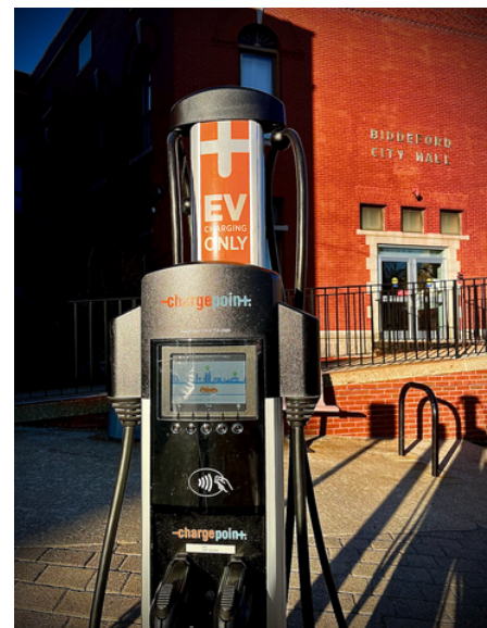
EV Charing Station. PhotoVoice Contest 2023 Entry.
