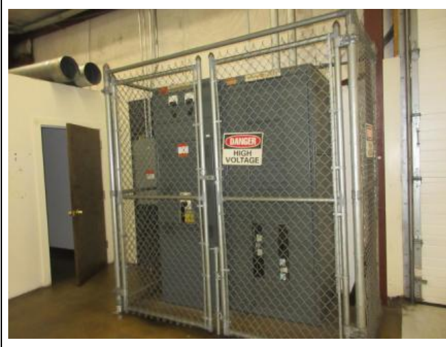
43) One of the main electrical entrances
