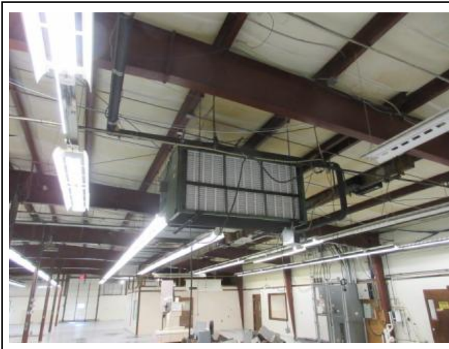
39) A heating unit in original section
