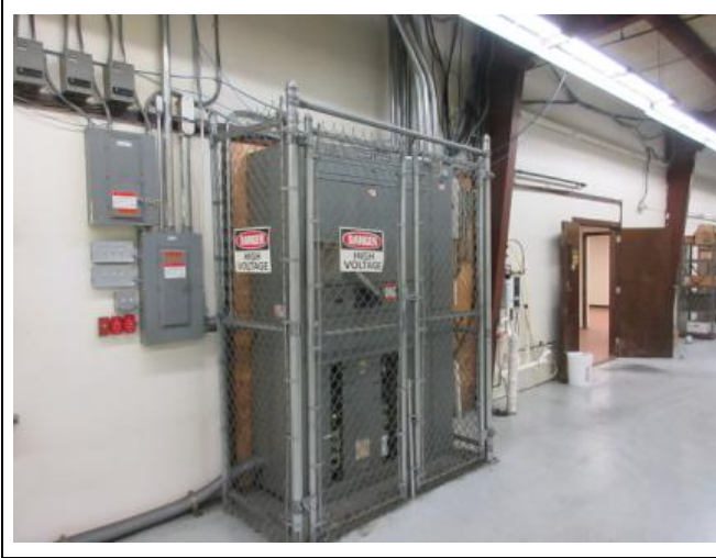
31) One of the main electrical entrances
