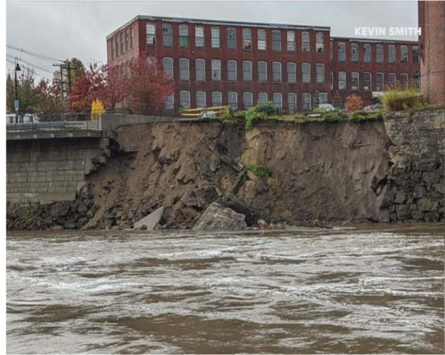
Failed Wall and Damaged MSE Wall
