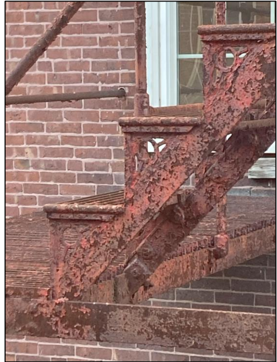
The fire escape is in poor repair, but the architectural detailing can still be seen.
