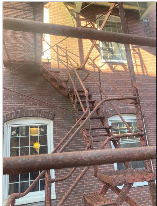
The escape is attached to the masonry in many places.
